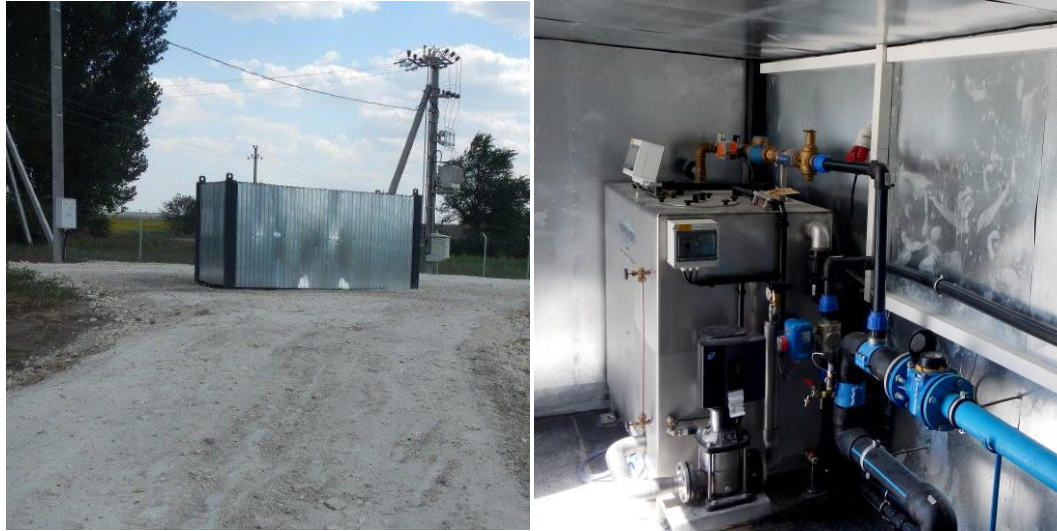
Figure 2: Housing for the in-situ system (left) and in-situ system equipment (steering unit, degassing tank and plumbing) (right) installed in Șerpeni, Moldova
